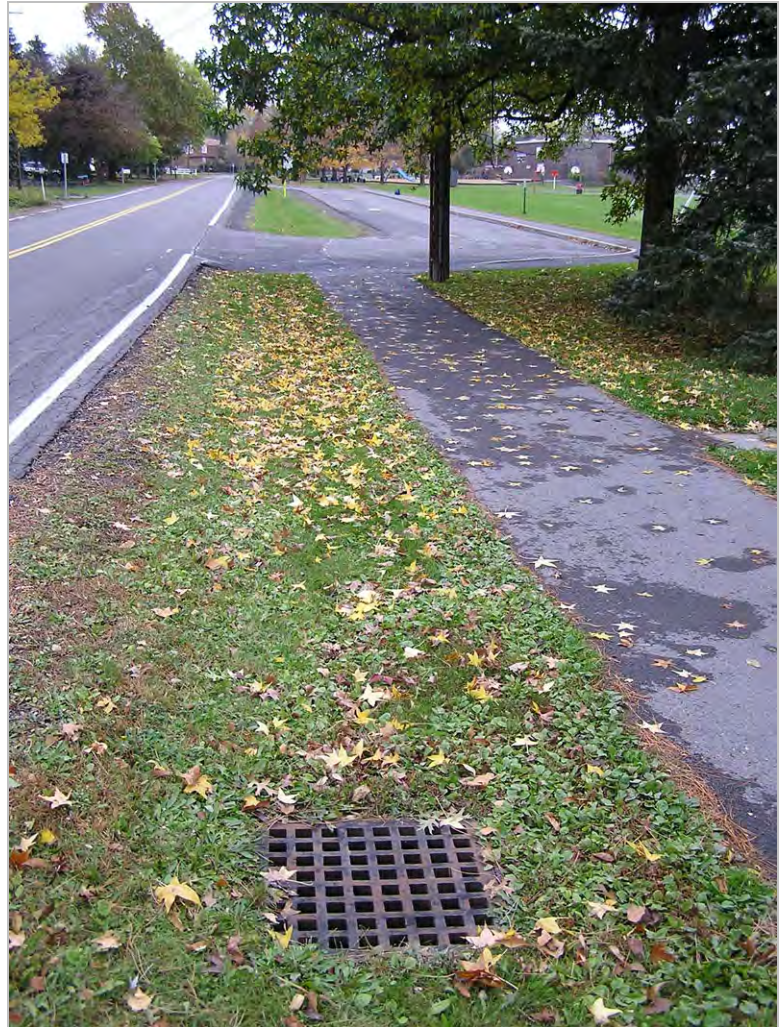
Stormwater inlet on Winthrop Drive, part of a larger drainage improvement project in Northeast Ithaca.
