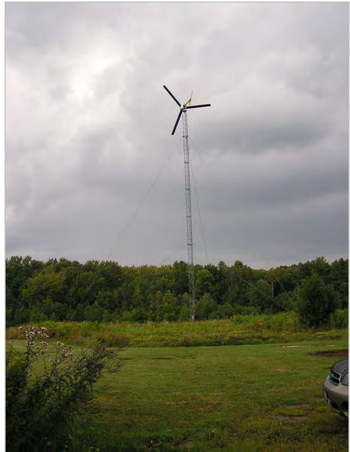
Residential wind turbine, Town of Ulysses
